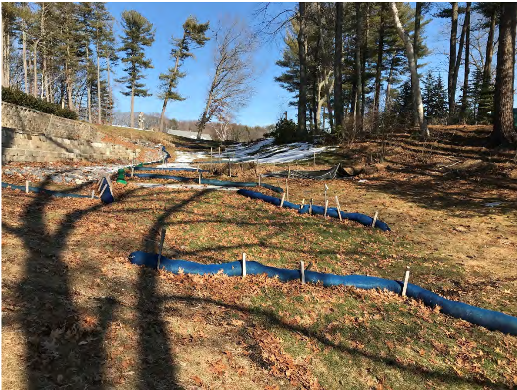
Fig 10: Slope below the manhole at Gundalow Landing/east side of the bay. Viewing east. (03-10-21)
