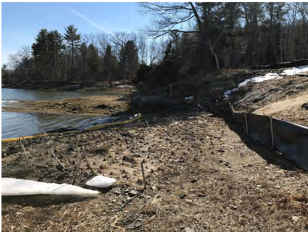
Fig 4: Toe of the slope and salt marsh restoration at the Eversource property/west side of the bay. Viewing south. (03-10-21)
